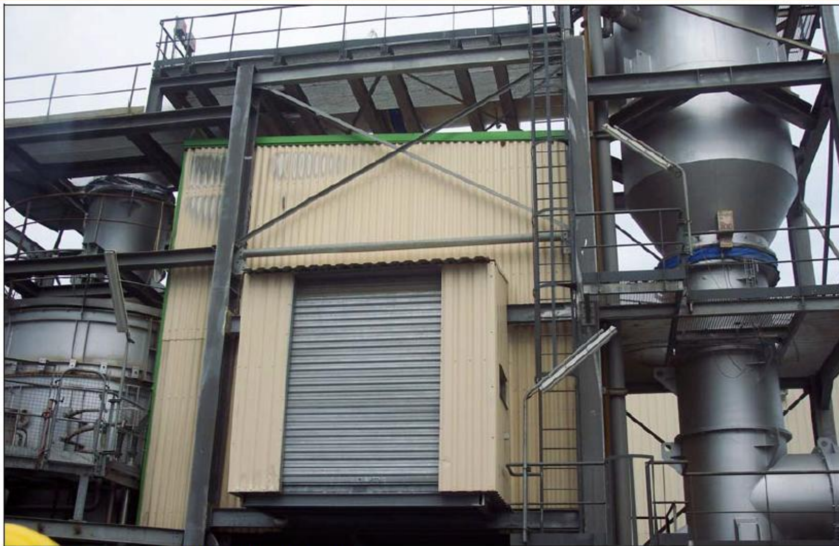
Photo Nr.7 Reactor filling hopper Plasma reactor on the left.
