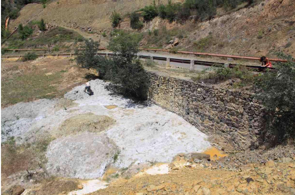
Covered tailing pond in Akhtala leaking.
